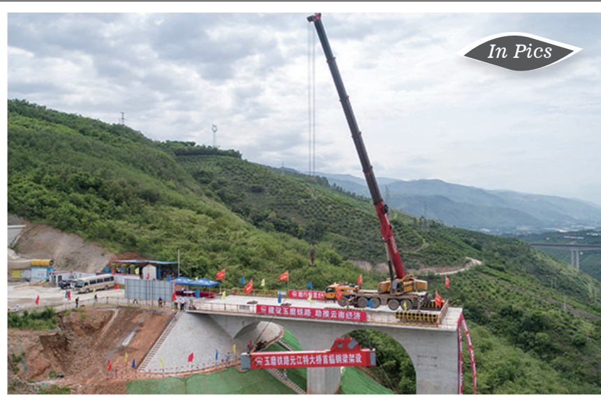
Builders began to lay the first steel truss complex on June 22 on the Yuanjiang Railway Bridge, in Yuanjiang County, Yuxi City of Yunnan Province, marking a new milestone in the construction of China-Laos railway. The 832.2-meter long bridge has 6 piers and its No. 3 pier is 154 meters tall, the tallest in the world. (Xinhua / Hu Chao)
